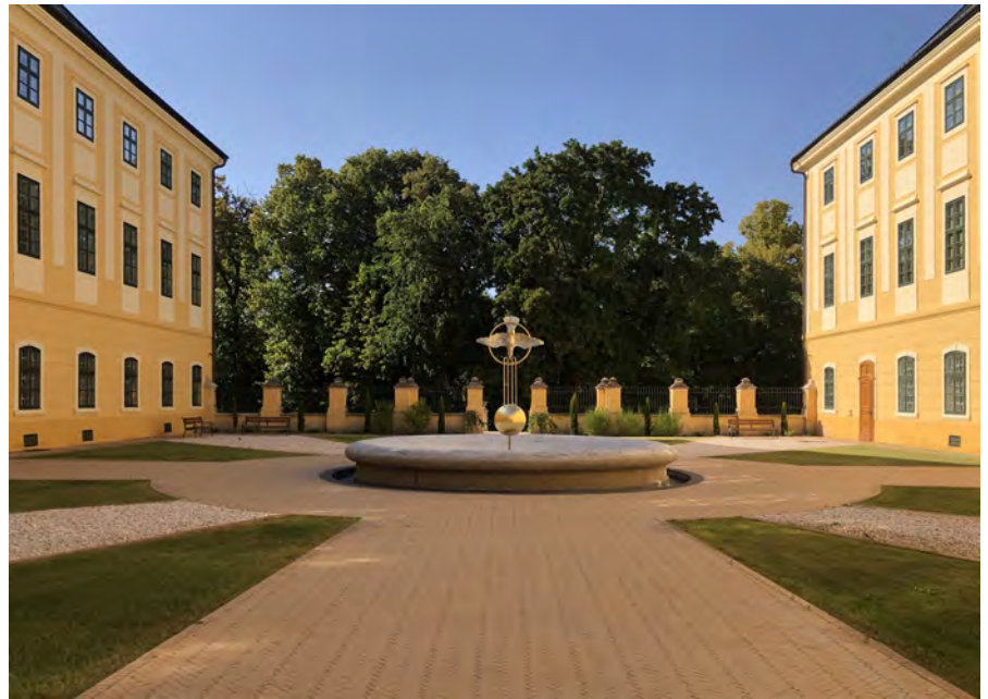
Figure 2 The inner courtyard of the Archbishop's Castle in Kalocsa with the fountain. Work in progress. Photo by Márta Vörös.
